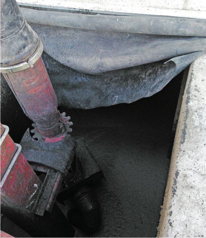
Figure 2. Example pump out curtain. Weight (PVC pipe with some gravel in it or a piece of metal) should be attached to the curtain to hold it at the manure surface.
